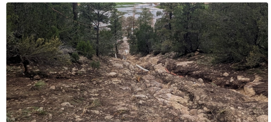
Where the water went. The scour channel runs from the tank site down to the school athletic fields.
