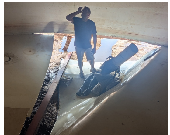
Inside the tank. The floor tore open at the seams and the whole bottom let go. The person is standing there for scale.
