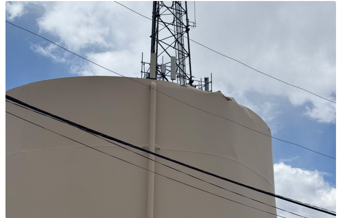
The top of a steel tank after a failure. A tank gives very little warning from the outside, which is exactly why the inspection interval matters.
