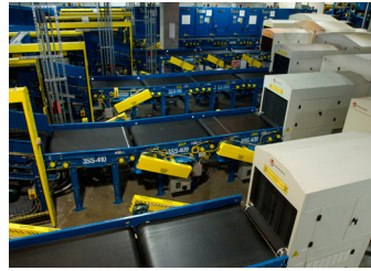
Baggage Handling Systems
