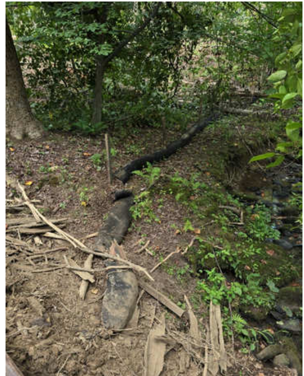
Example of Compost Filter Sock (CFS) not properly installed on a logging site
