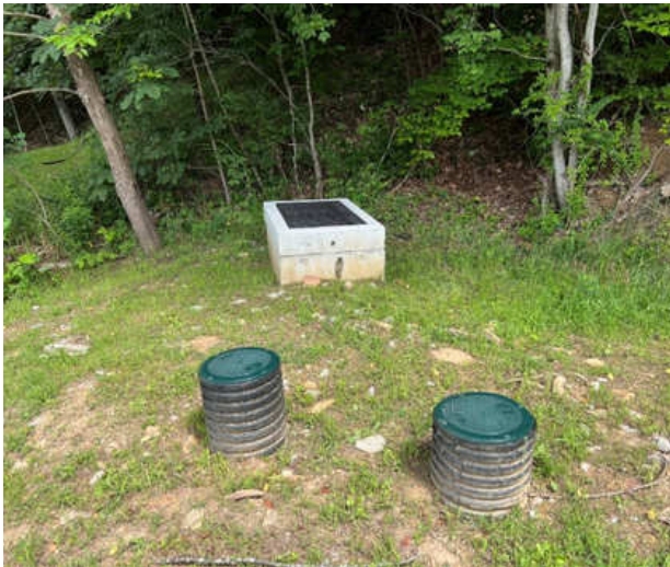
After - Flow splitting box
