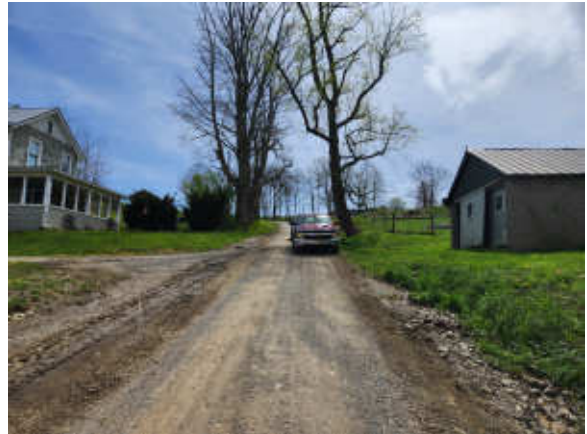
Before - steep, deep ditch road
