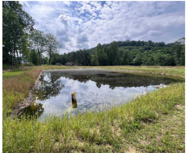
After - treatment wetland
