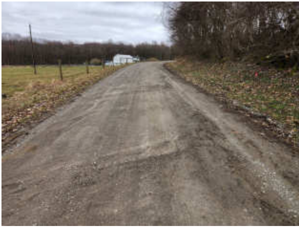
Before - deep ditch, low drainage road
