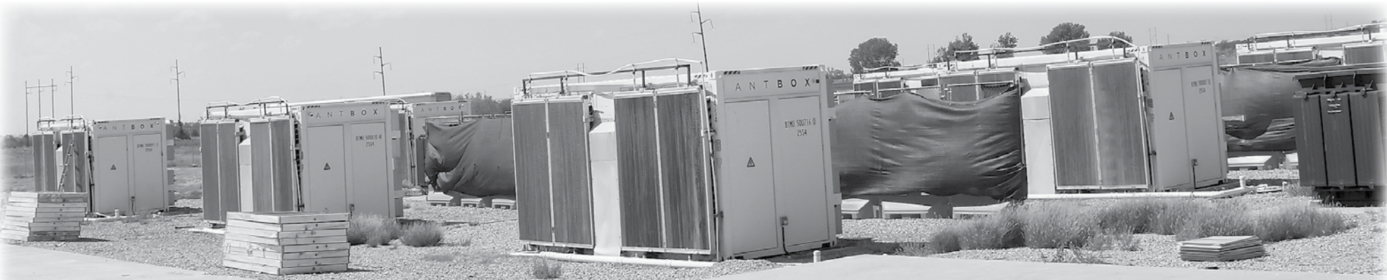
Bitcoin mining center operating illegally in El Reno, Okla., was brought to light by a damaged fire hydrant on the property that ended up leaking over 3.8 million gallons of water.
