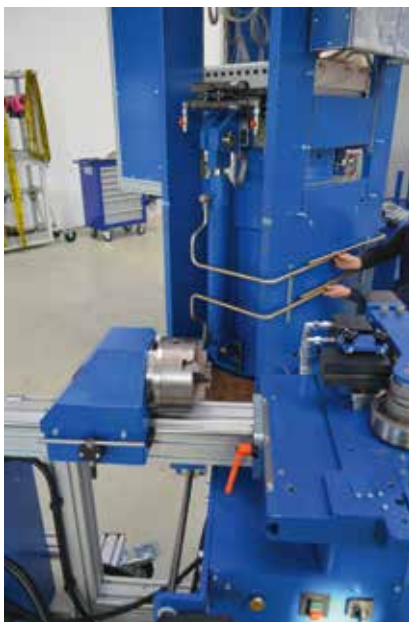
Tubing fitted directly to plant and on-board calculations
