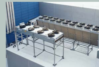
Picture of the cooling towers of the new process water cooler and recycler
