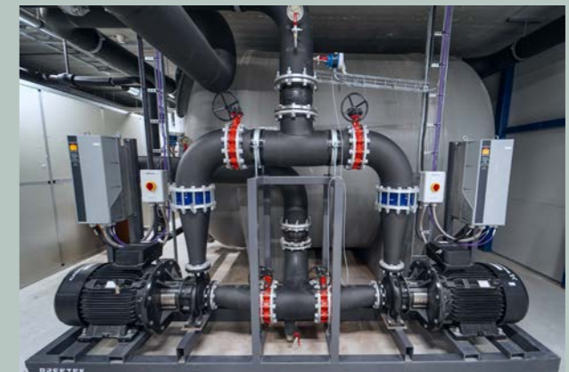
Picture of our new process water recycling plant
