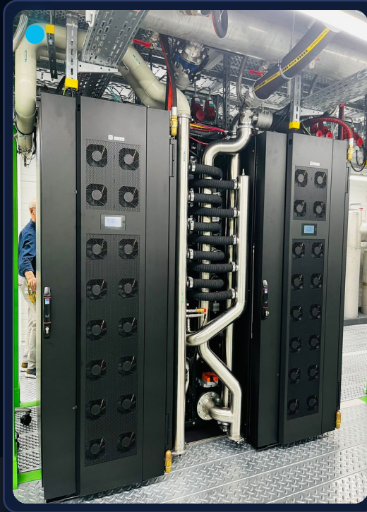
Cooling & liquid infrastructure
