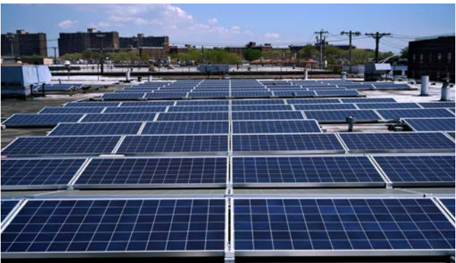
1.05 MW of PV, ~1.5 GWh/yr
