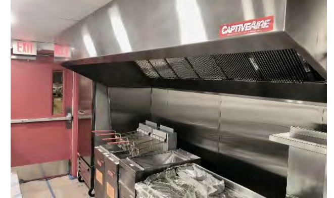
Kitchen Hood Controls
