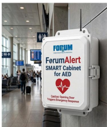
ForumAlert Smart Cabinet for AED — installed at airport terminal gate
