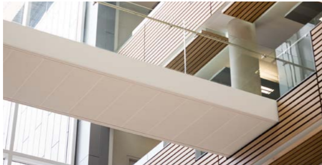
MBS SAS205 System: Corridor Ceiling
