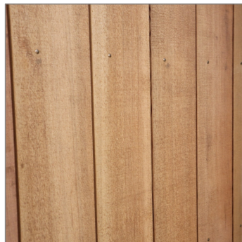
Natural cladding - Selected Vertical Cedar w/board cladding
