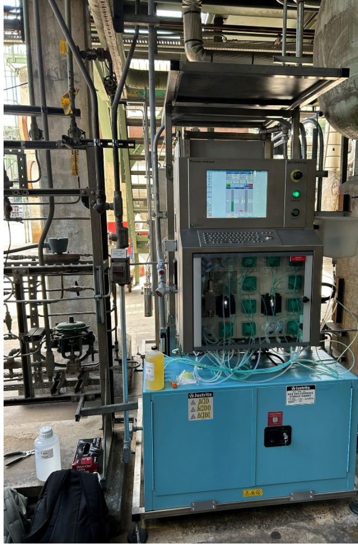
FIGURE 8. 2045 TI EX PROCESS ANALYZER INSTALLATION AT A LARGE WEST COAST REFINERY.
