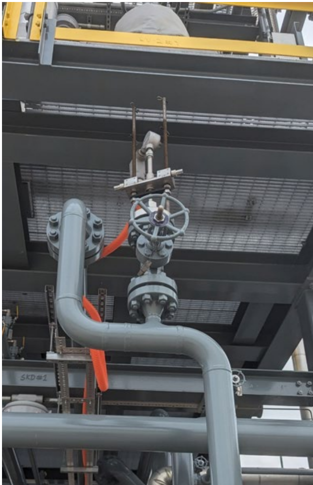
FIGURE 6. INADEQUATE INSTALLATION DESIGN PREVENTING PROPER MAINTENANCE
