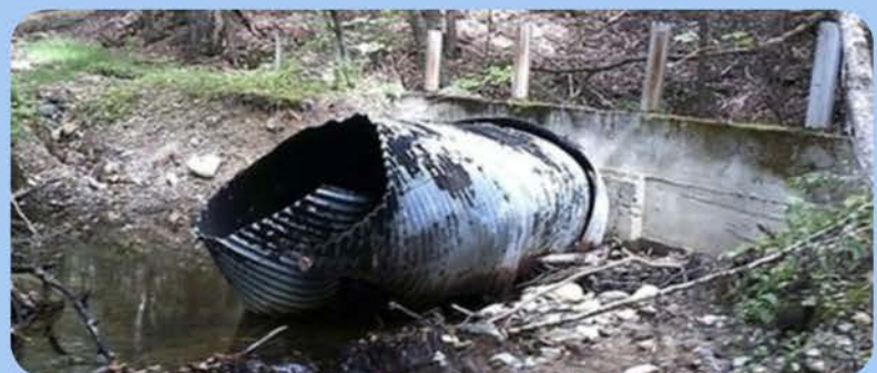
Washed-out culvert on Ratlum Brook
