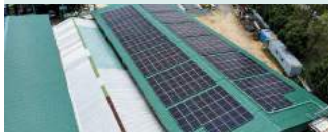
Solar panels at Kertih Workshop located in Kertih, Terengganu
