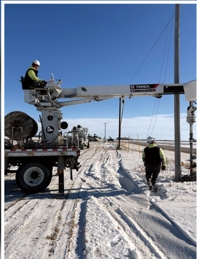
Connor Eidsmoe (left) and Chad Johnson removing old poles from a line rebuild in Ross Township.
