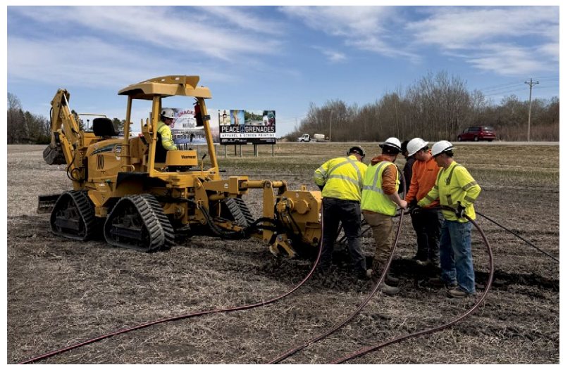
REC and Northstream Fiber crews working together to install three-phase wire and fiber for the Highway 11 road construction project
