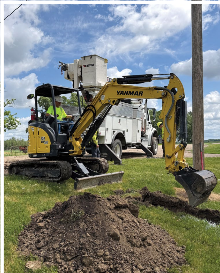
Chad Nelson, line crew foreman, works on an overhead-to-underground line conversion in Whiteford Township.
