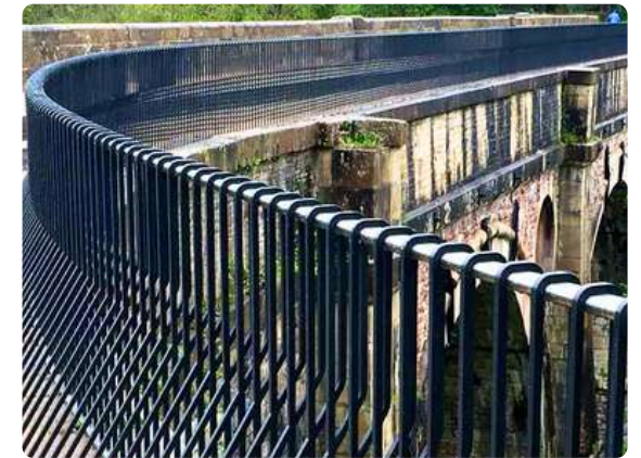
Marple Aqueduct, Bisca Architects (flat-sided oval tube, stainless steel 316L, 62 x 31 x 3mm)
