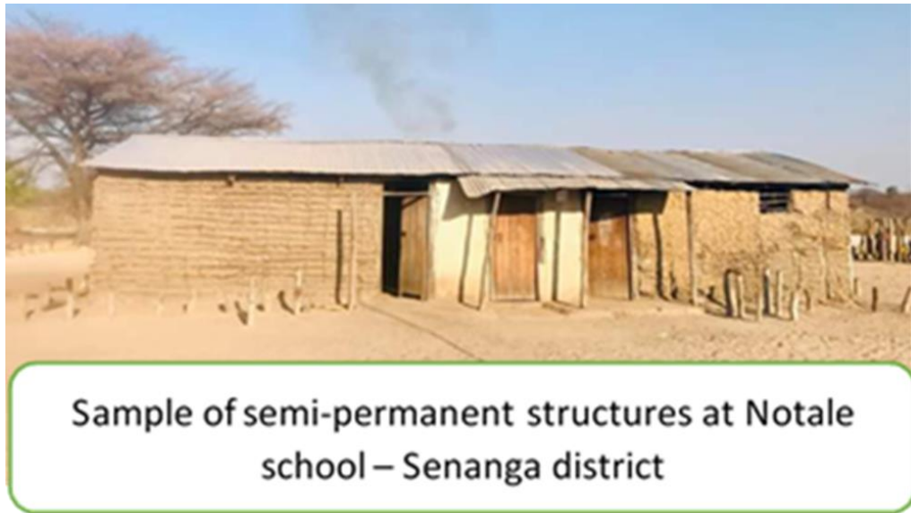
FIGURE 15: PICTURE SHOWING STATUS OF POLE AND MAD CLASSROOMS
