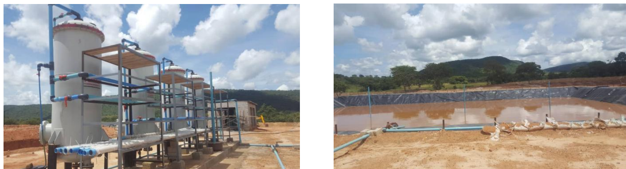
Figure 8: Infrastructure at Gold Processing Plant
