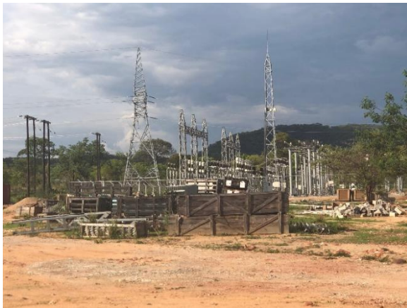
Figure 15: 132/33kV Mpanshya ZESCO Substation
