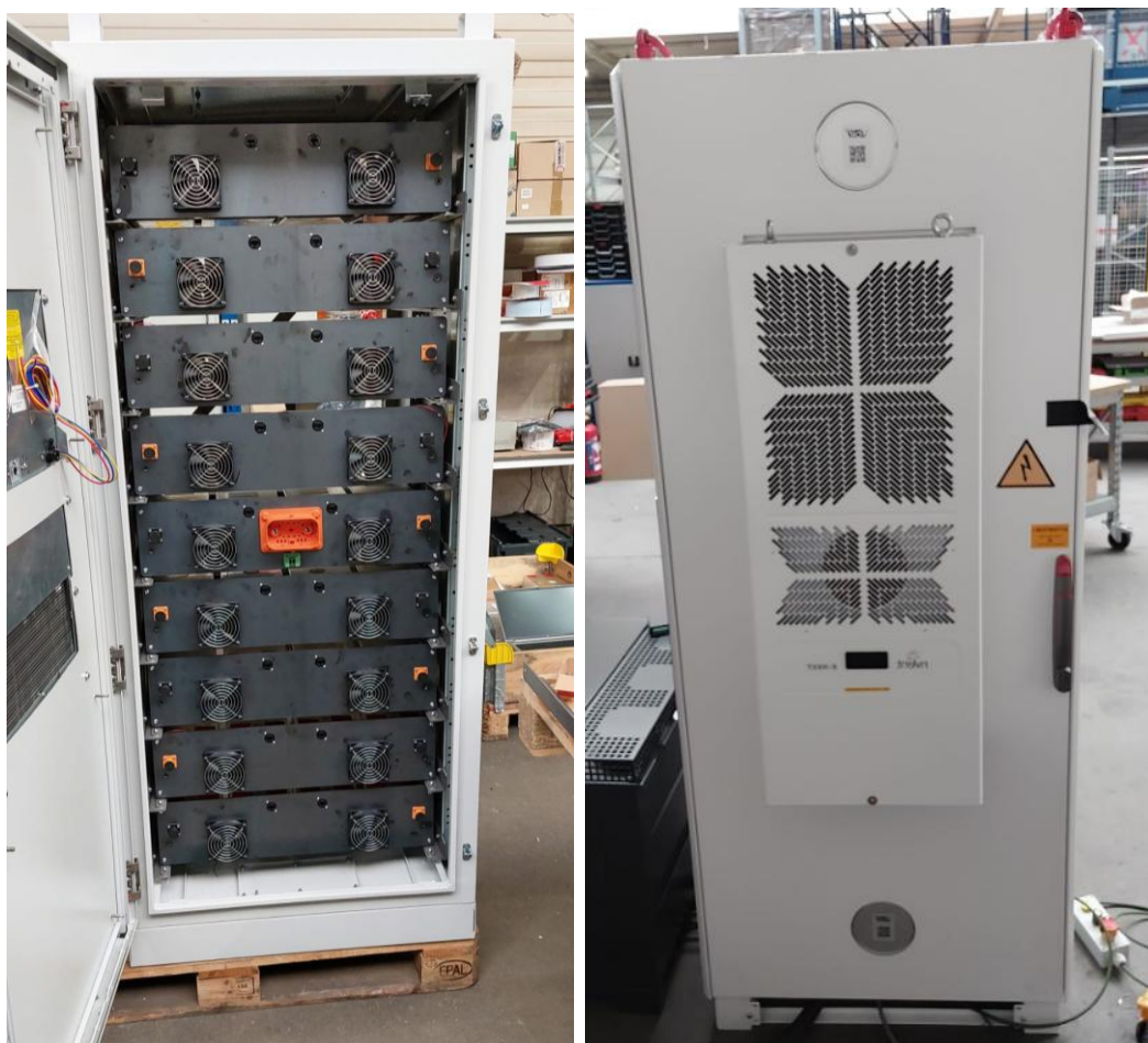
Figure 18. The BESS cabinet ready to be tested
