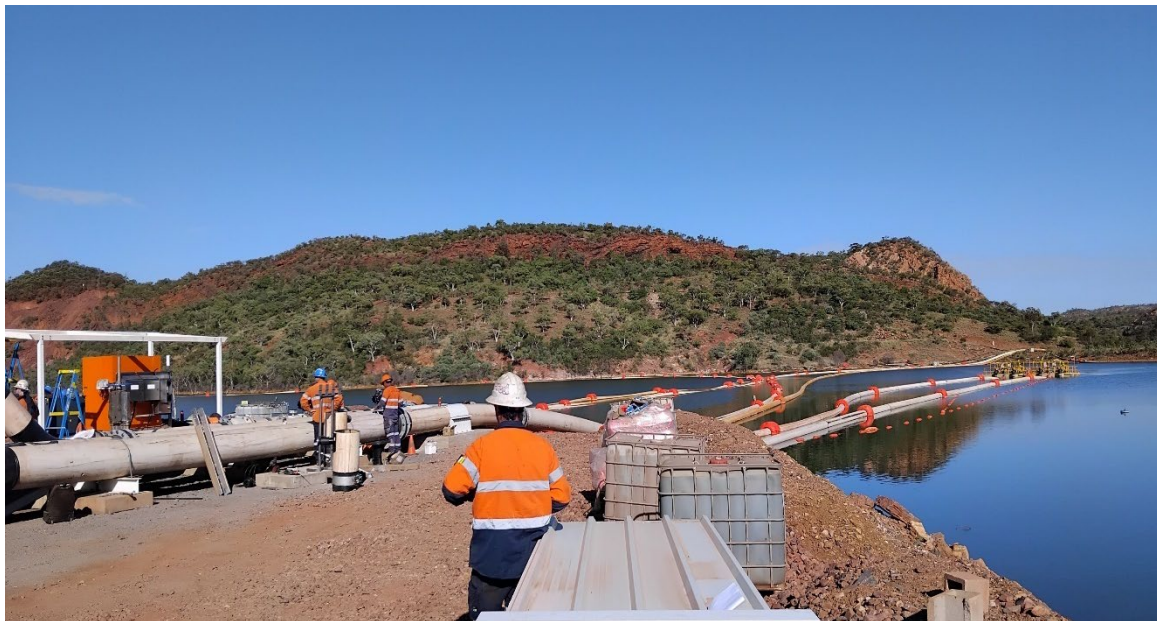
Figure 9: Completed MCD bulk treatment and release system (May 2024)
