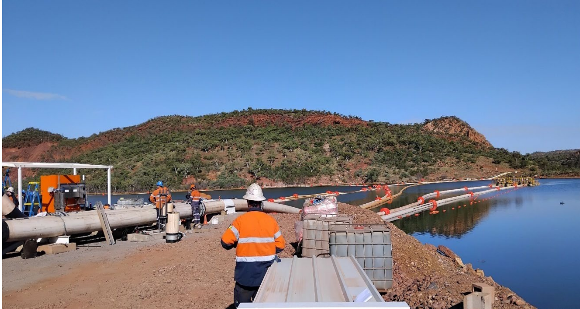
Figure 19: Completed MCD bulk treatment and release system (May 2024)
