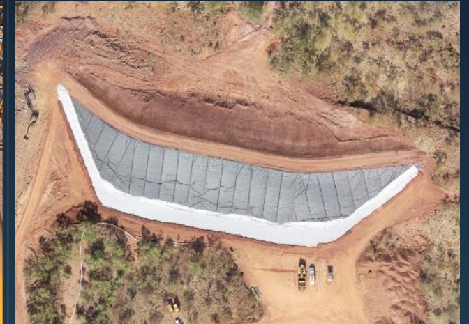
Enhanced water diversion infrastructure
