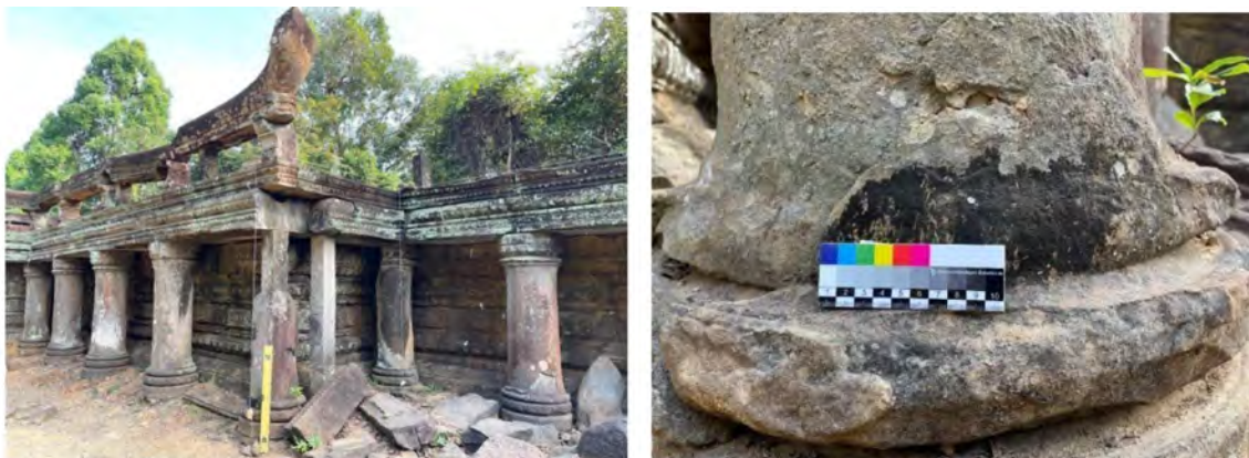
Figure 6.12: Stone damages Increased humidity, temperature (Photo: HIN Chandara 2024)
