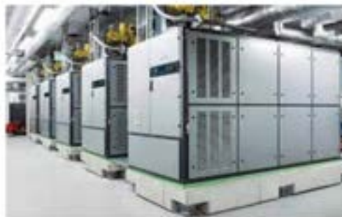
Combined heat & power system implementation
