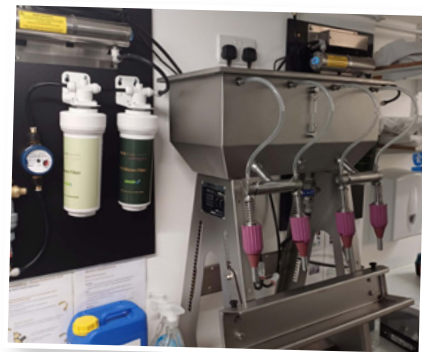
ECOPURE Water system at Crowne Plaza Nottingham
