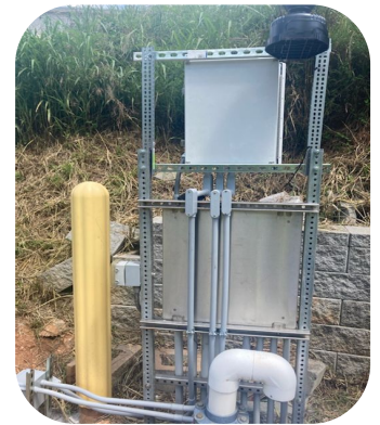
CMAC control panel and monitoring station
