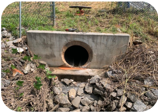
Passive outlet structure
