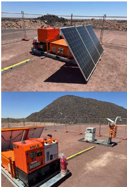
Figure 25: RocketDNA SolarSkid hybrid off-grid Dock solution
