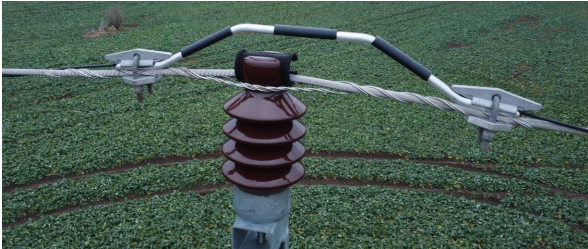
Fig. 5 – Detail of the transition over insulator
