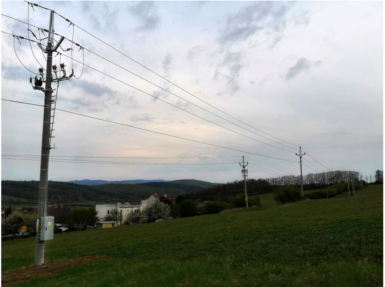
Fig. 1 – All-dielectric self-supporting cable
