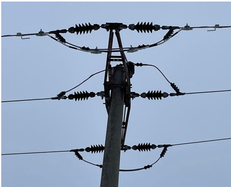
Fig. 8 – The arcing horns on the line
