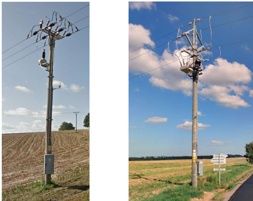
Figure 1: On the left: switch, on the right: recloser
