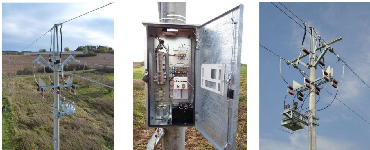
Figure 2: Detail view of the recloser
