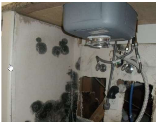
Visible Mold Under Cabinets
