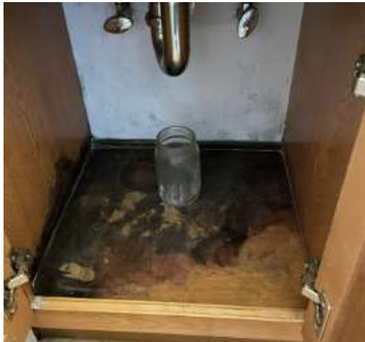
Dark Staining under Cabinets
