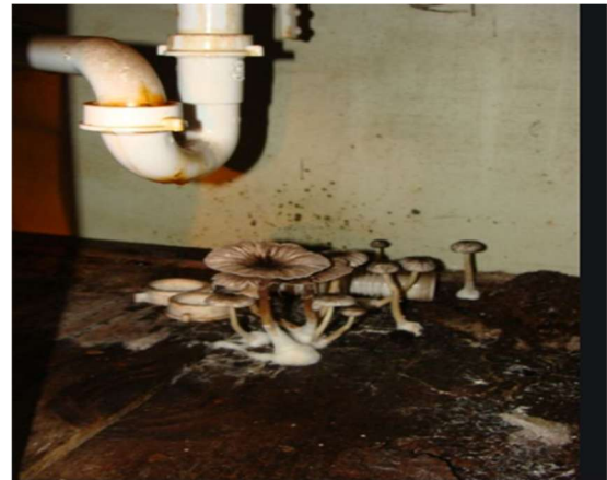
Long-Term Damage Under Kitchen Cabinets
