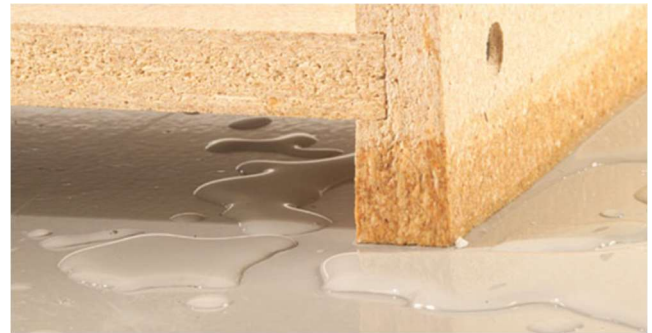
Swollen Particleboard Cabinets
