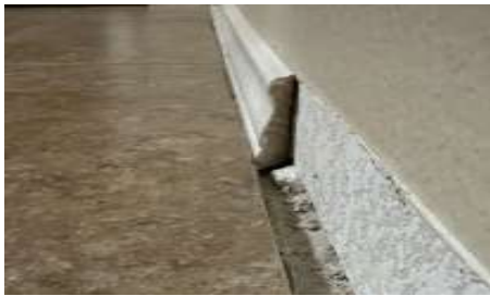
Tile grouted up to baseboard causing it to be difficult to remove without cracking the tile.
