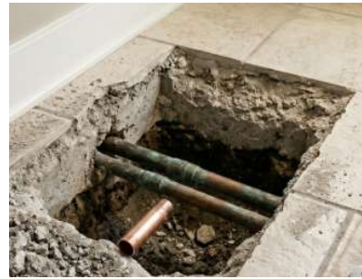
Slab leak under ceramic tile
