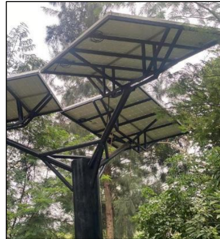
Photo 11: One of the solar panel units in NUWEP used for lighting.
