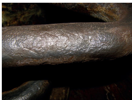
Figure 5. Corroded external tube surface
