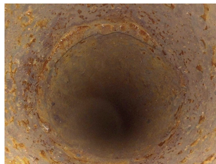
Figure 4. Internal boiler tube corrosion.
