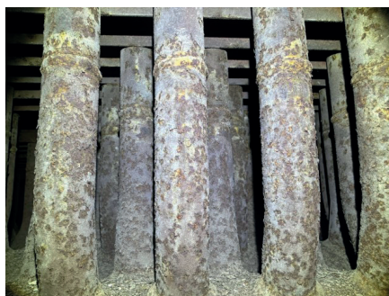
Figure 1. External boiler tube corrosion
