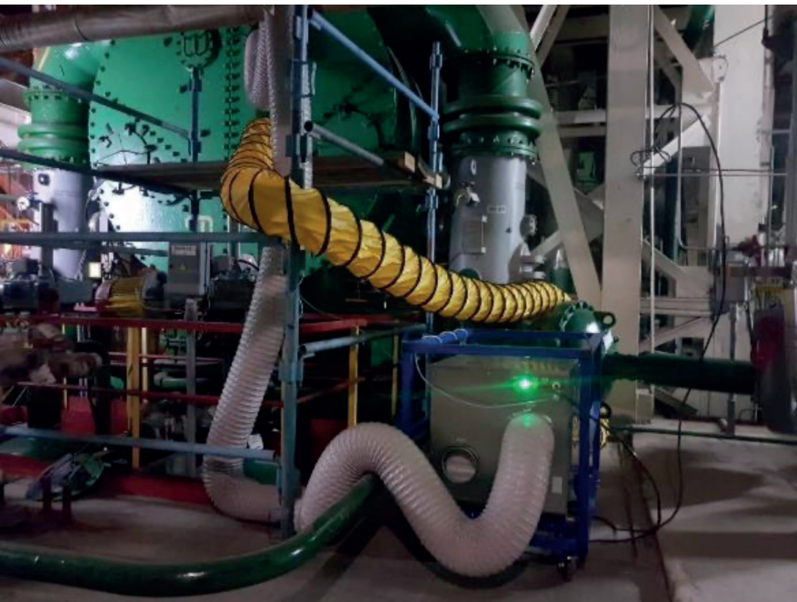
Figure 7. Dehumidifier ducting to steam turbine for preservation. Photo: Tetra Engineering
