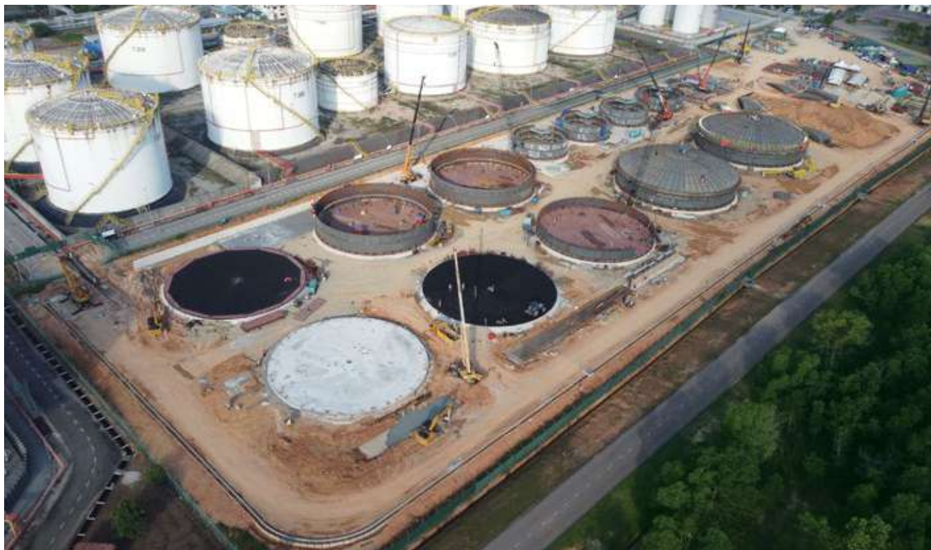
The second phase of renewable fuel storage expansion, DIALOG Terminals Langsat
