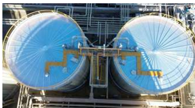
Tank turnarounds for Puma Energy, Townsville, Australia
