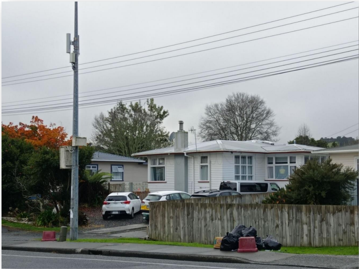
Onerahi (Whangārei) 4G mini cell tower directly outside residential home – photo taken by the author
