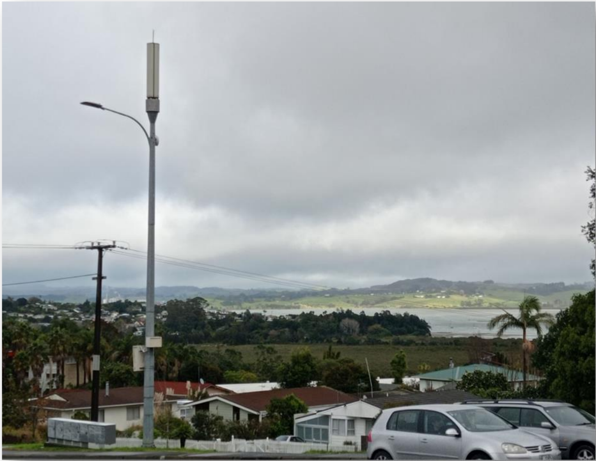
4G mobile cell tower outside homes (Onerahi, Whangārei) – photo by author
