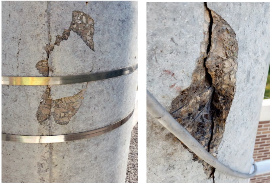
Figure 6-6: Spalls (left), major cracking and spalls (right)
