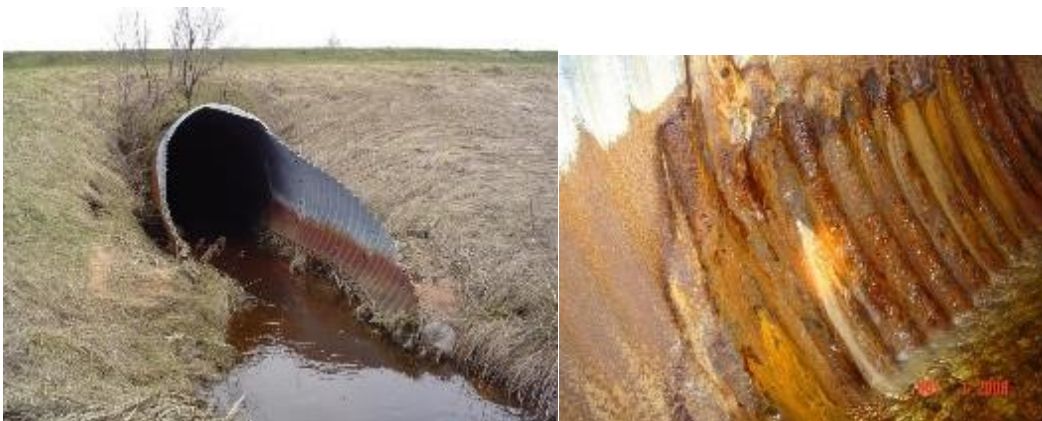
Figure 2-36: Loss of protective coatings contributing to corrosion
