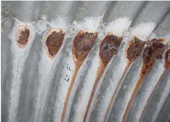
Figure 2-35: Corrosion of a metal culvert
