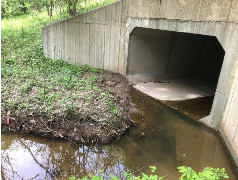
Figure 2-14: Stream channel poor horizontal alignment
