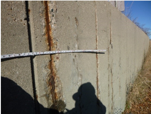
Figure 3-10: Corroded wall reinforcing
