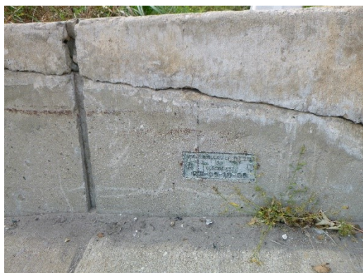
Figure 3-9: Horizontal structural cracking
