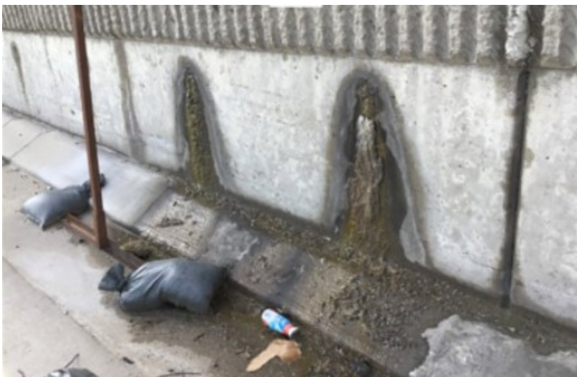
Figure 3-13: Retaining wall concrete abrasion
