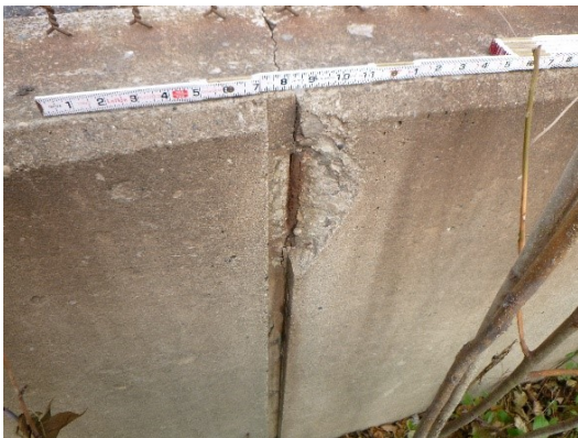
Figure 3-11: Concrete spall with corroded reinforcing
