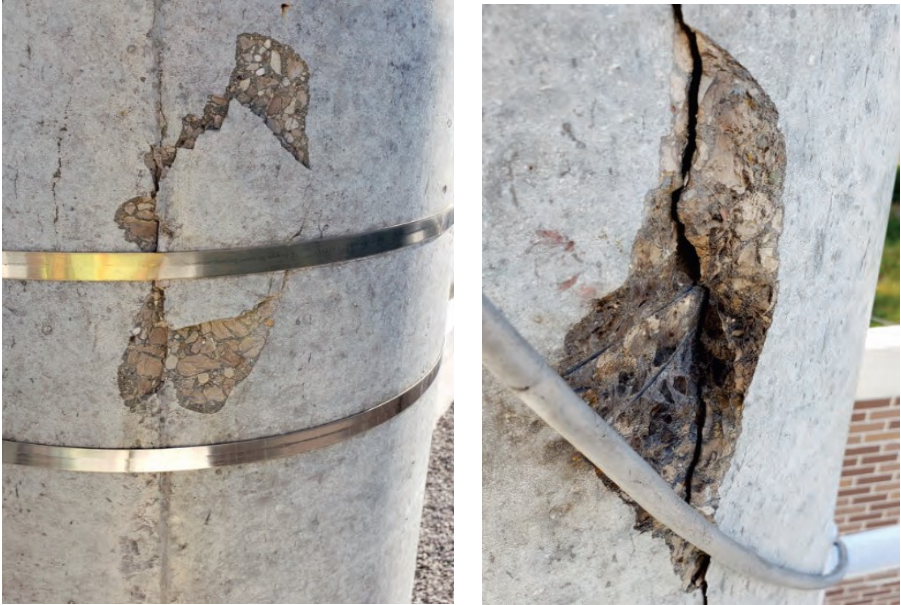
Figure 6-6: Spalls (left), major cracking and spalls (right)
