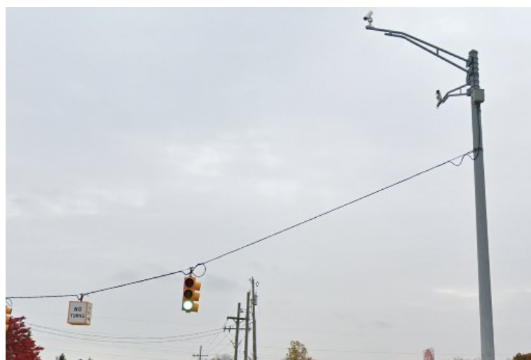
Figure 7-20: Cameras mounted on luminaire truss arms
