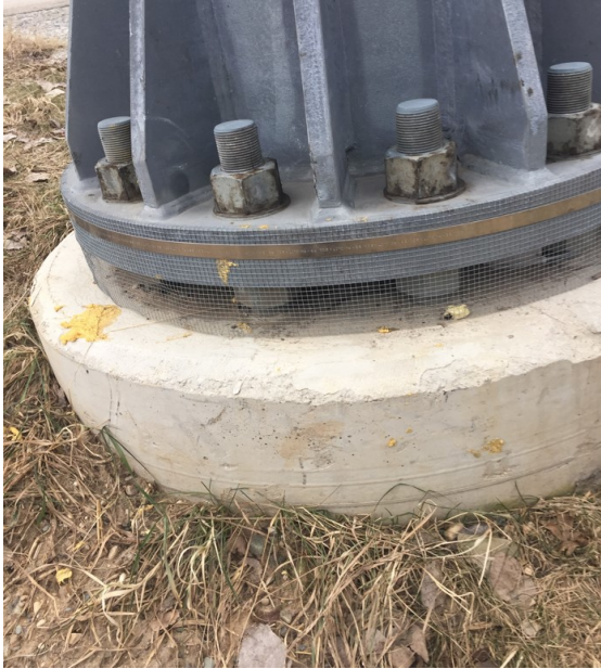
Figure 10-4: DMS support structure foundation, minor spalling
