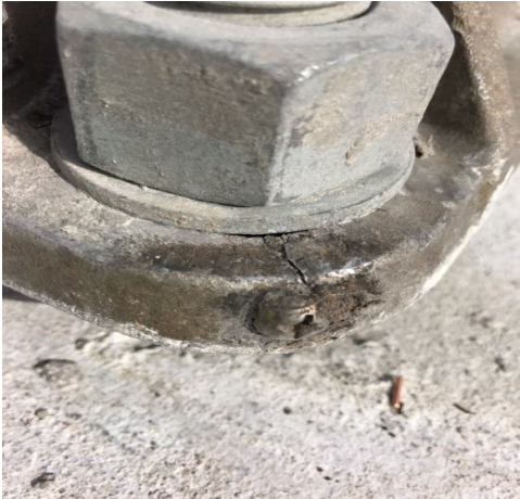
Figure 11-15: Non-frangible pole structure base plate crack
