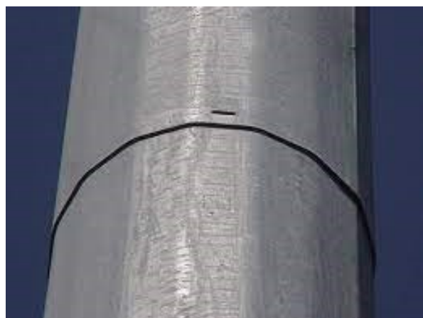
Figure 12-7: HMLT pole splice
