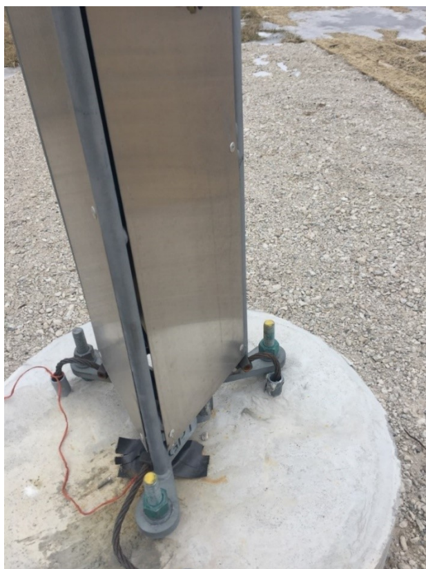
Figure 14-6: ESS tower base plate
